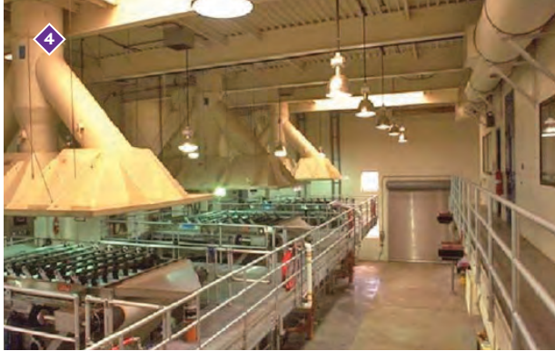
Biosolids Dewatering Belt Filter Presses
